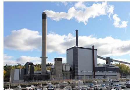
Flue gas scrubber for the Naistenlahti plant, 10 MEUR
