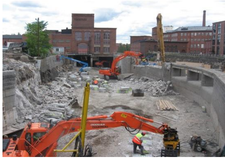
Renewal of the hydropower plants at the Tammerkoski rapids, 2010–2012
